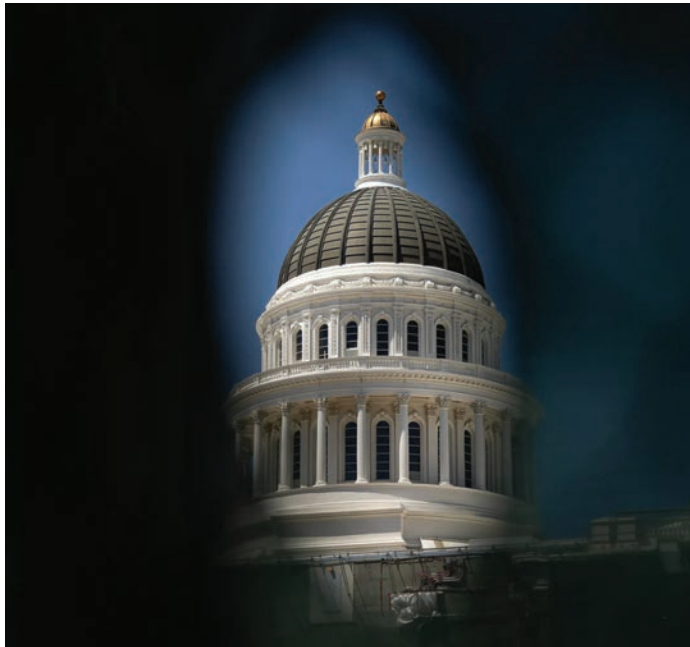
Construction of the annex at the state Capitol in Sacramento on April 29, 2024. Photo by Miguel Gutierrez Jr., CalMatters
